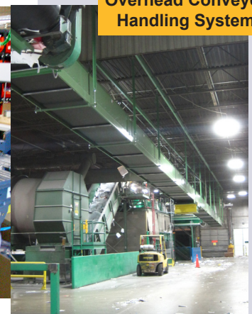
Custom Package Handling System
