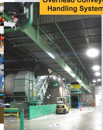
Custom Package Handling System
